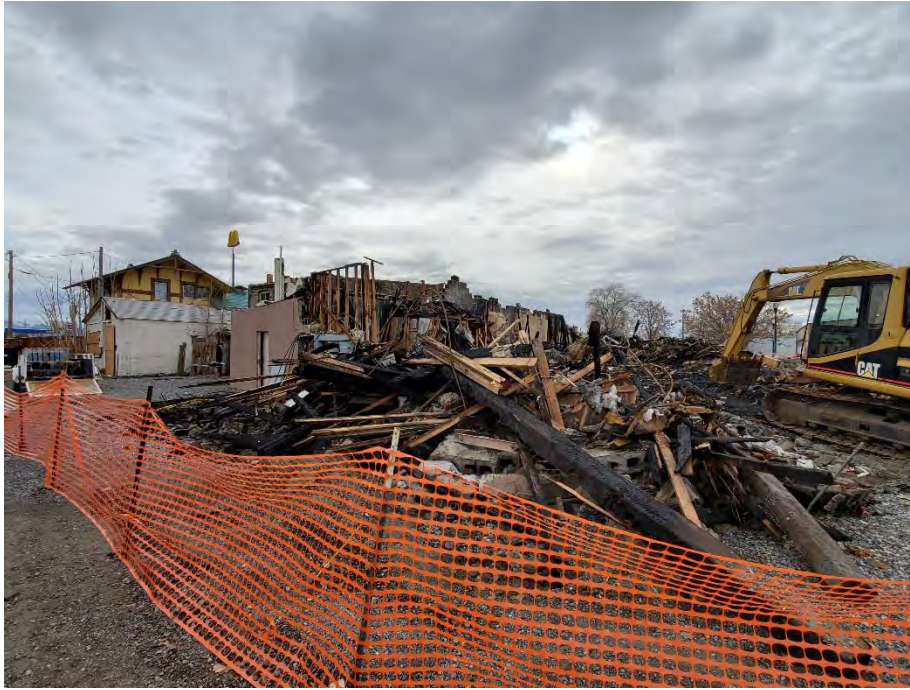
Photograph 11: View of rubble on southeastern adjoining property.
