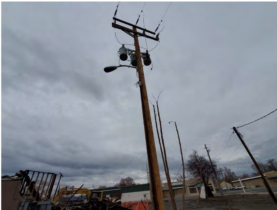
Photograph 14: View of three pole-mounted transformers.
