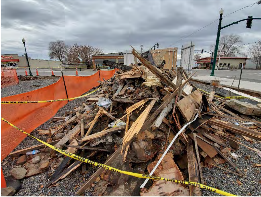
Photograph 15: Direct view of rubble on the Property.
