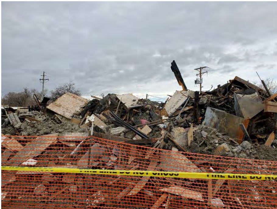
Photograph 4: View of rubble on the Property.
