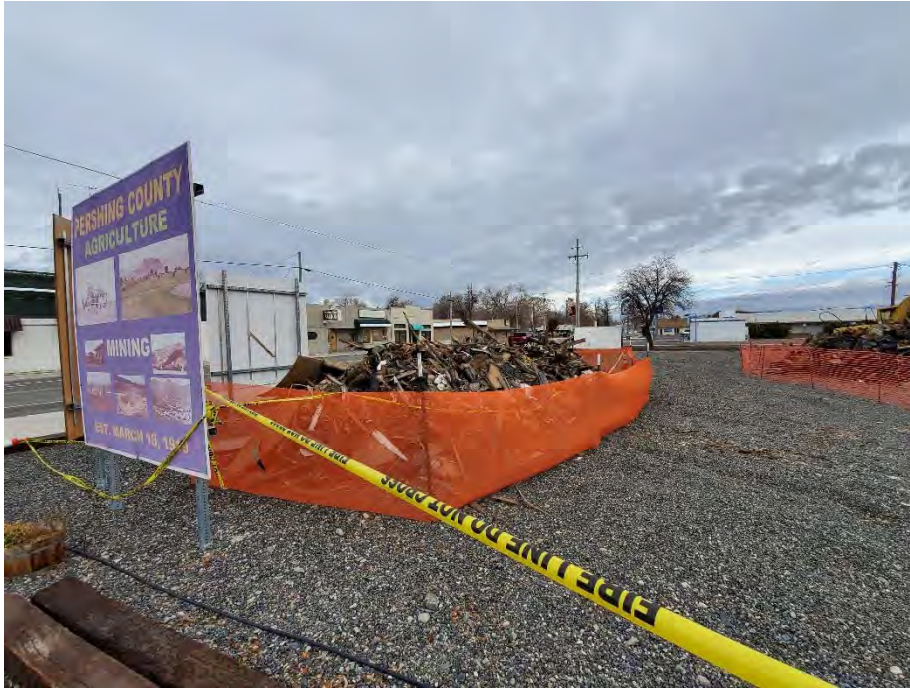
Photograph 5: General view of the pile of rubble located on the northwestern adjoining property.
