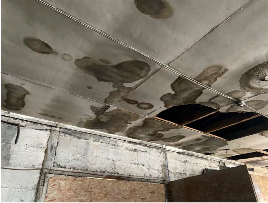
Photograph 25: View of suspected fungal growth on ceiling.
