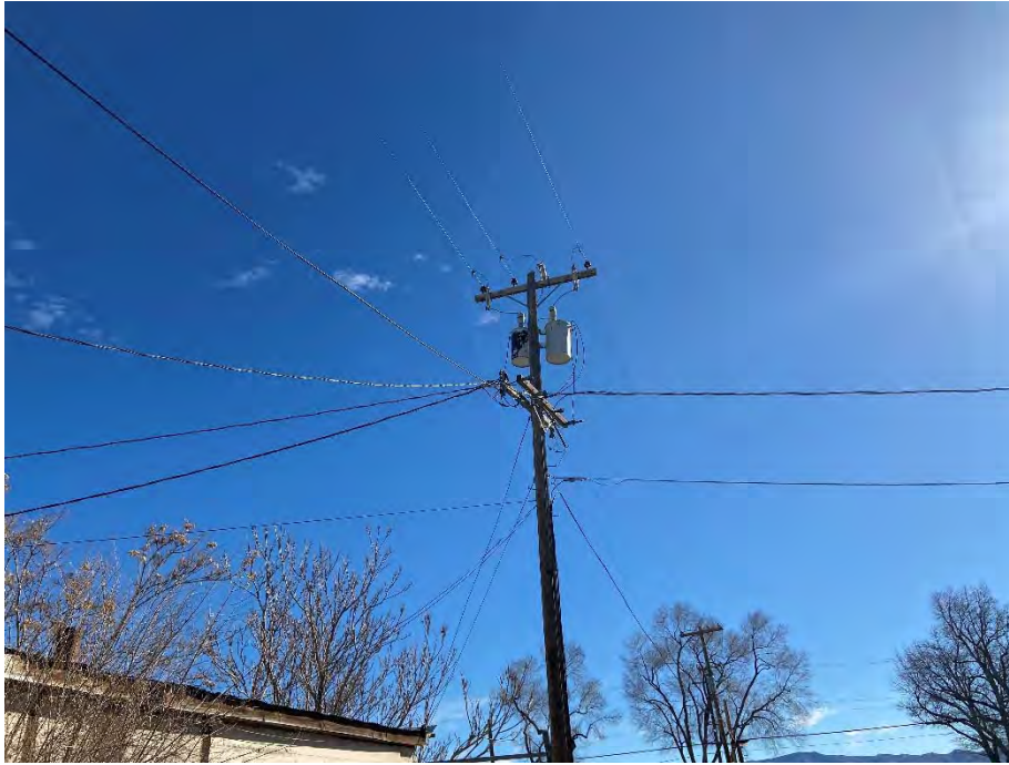
Photograph 17: View of (2) pole-mounted transformers.
