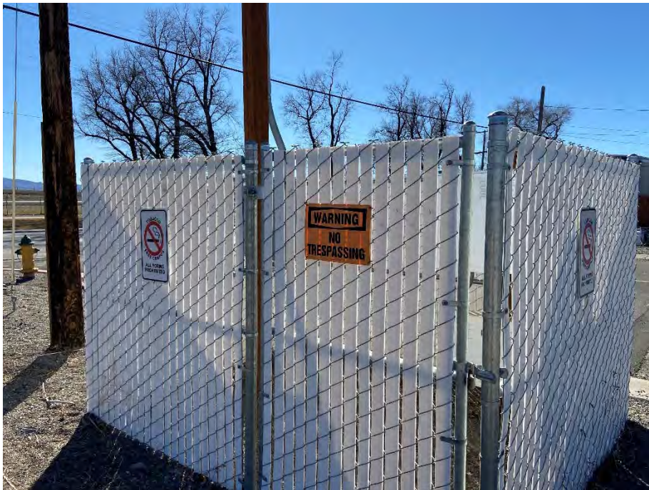
Photograph 18: View of electrical access on the southeastern portion of the Property.
