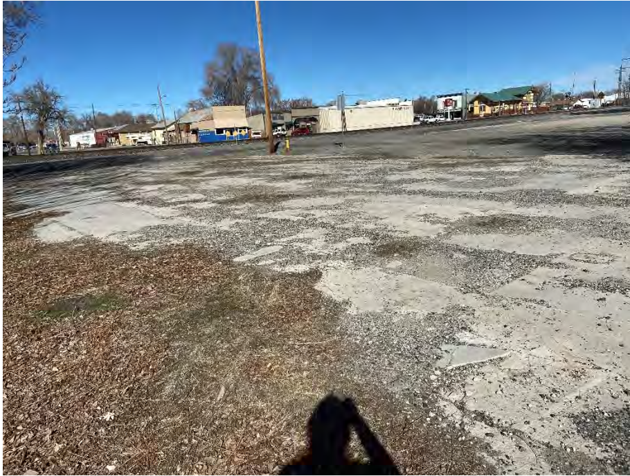
Photograph 13: View of the remnant building foundation on the northern portion of the Property.
