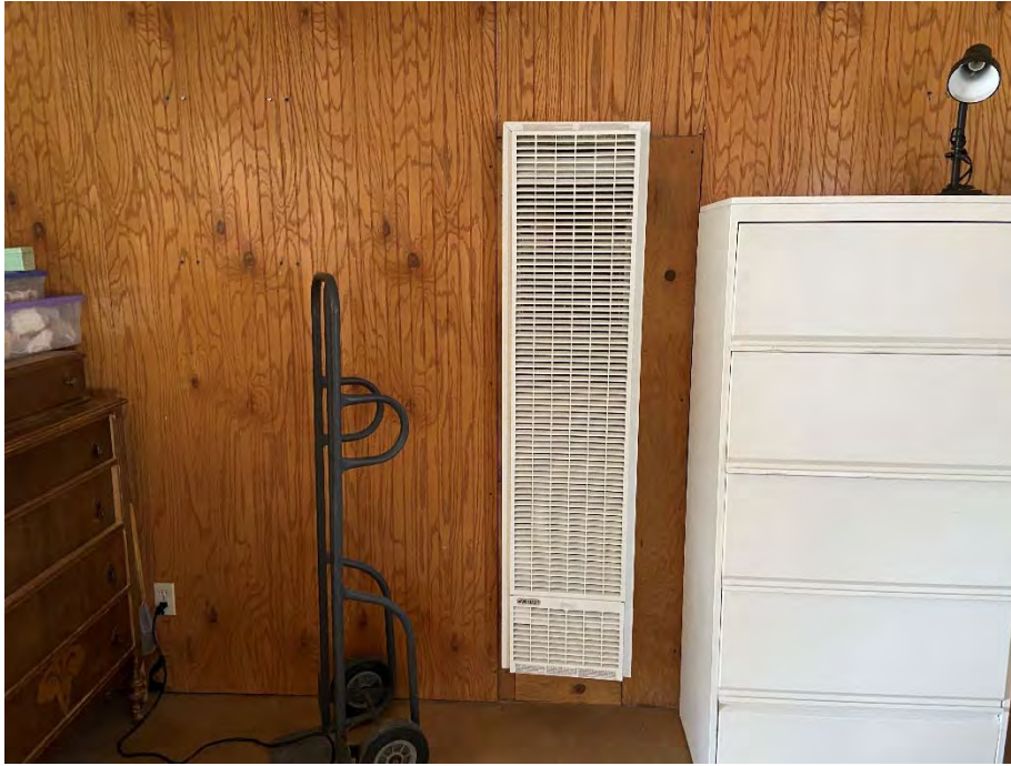
Photograph 15: View of heating unit in the larger residential unit.
