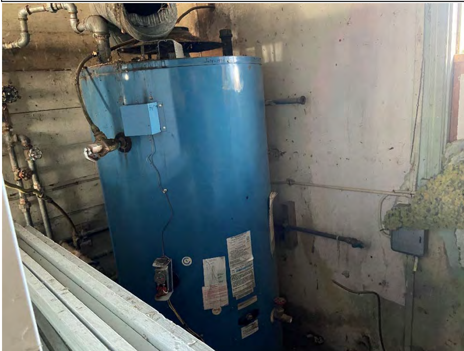
Photograph 10: View of central water heater located in the maintenance area of the motel building.
