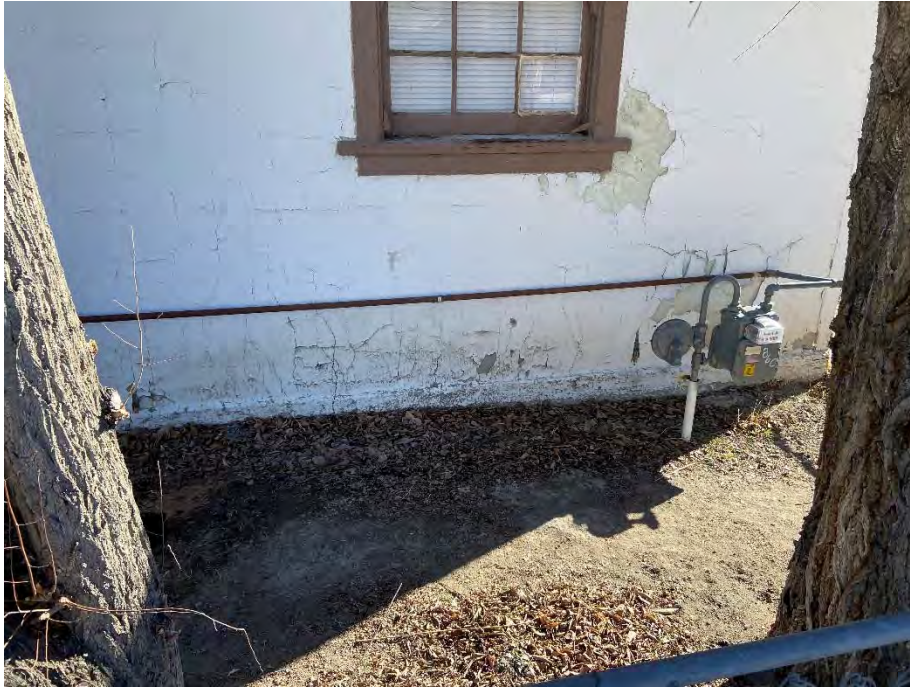
Photograph 13: View of natural gas line connected to the larger residential building.
