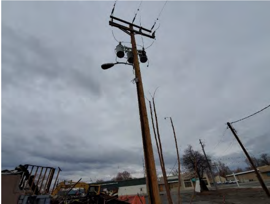
Photograph 9: View of pole-mounted transformers to the north of the Property.
