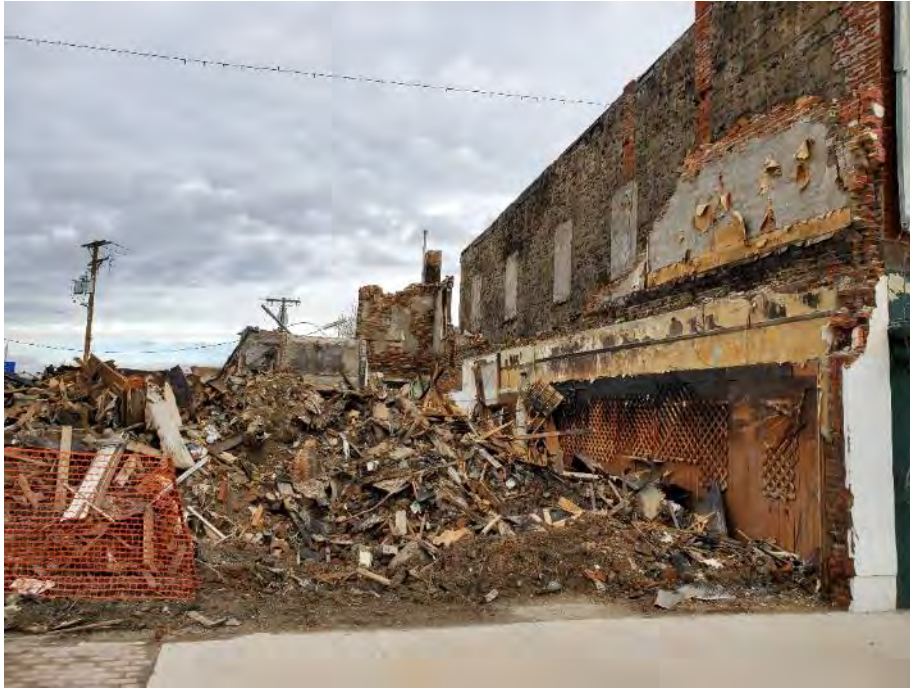
Photograph 1: View of the Property with rubble piles.
