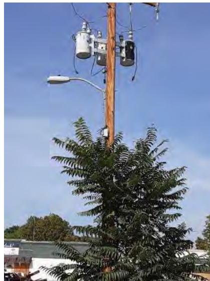
Photograph 8: View of pole-mounted transformers on the Property.
