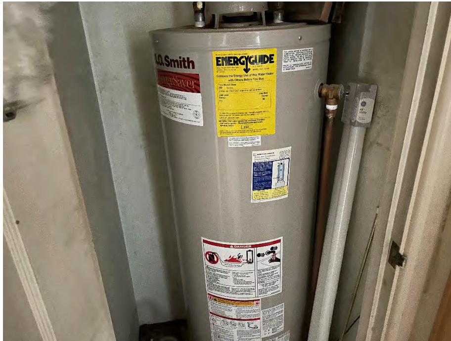
Photograph 9: View of the water heater.
