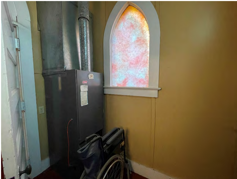
Photograph 12: View of the furnace in the church building.
