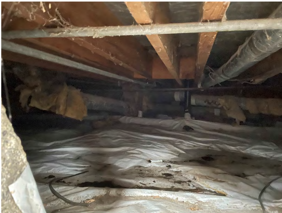
Photograph 14: View of radon vapor barrier located beneath the residential portion of the Property.
