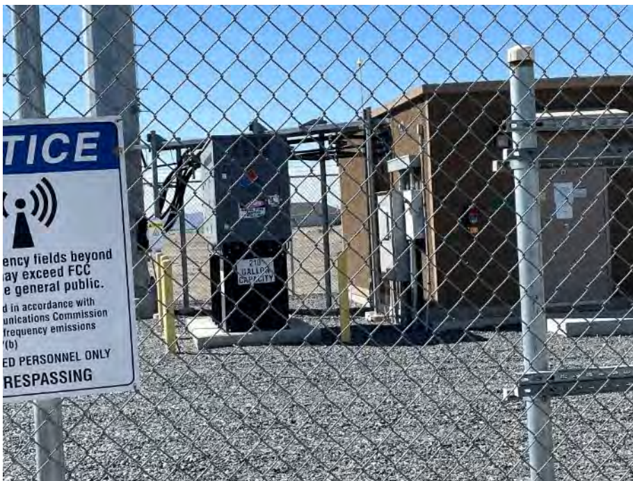
Photograph 14: View of the emergency generator located adjacent to the cell tower.
