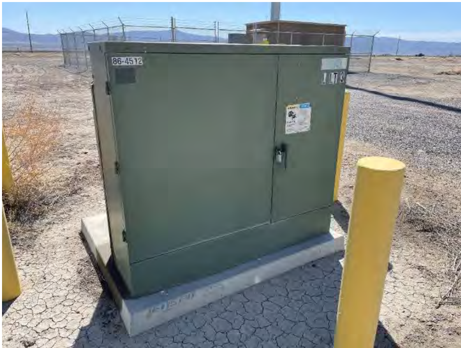
Photograph 12: View of the pad-mounted transformer located on the northern portion of the Property.
