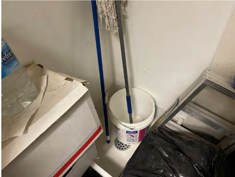
Photograph 29: View of the floor drain inside a utility closet in the Nevada Highway Patrol tenant space.
