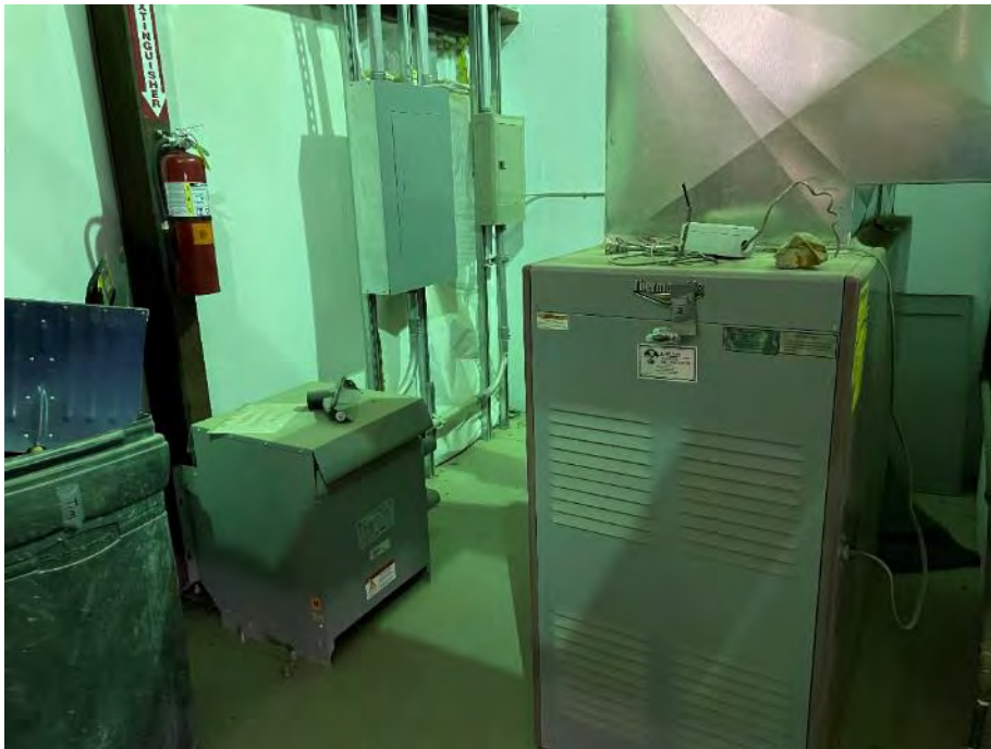
Photograph 8: View of the natural gas/electric furnace inside the warehouse building.
